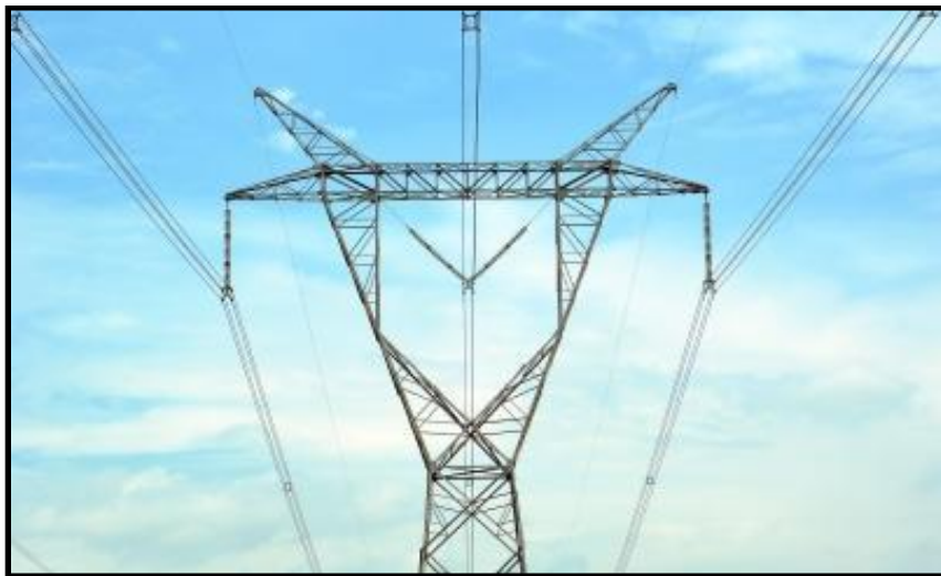
Figure 4. High-Voltage Power Transmission Tower and Cable [14]
