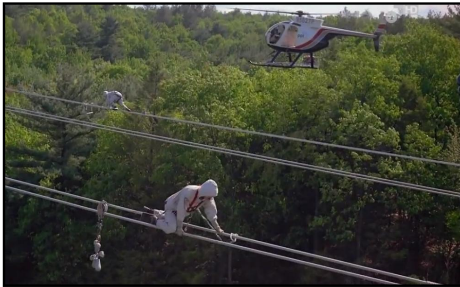
Figure 6. Crawling along High-Voltage Power Transmission Cables for Inspection (A still image from video) [16]
