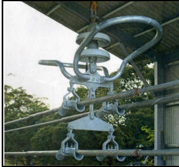
Figure 13. Suspender Clamps Holding the Power Transmission Cables [20]
